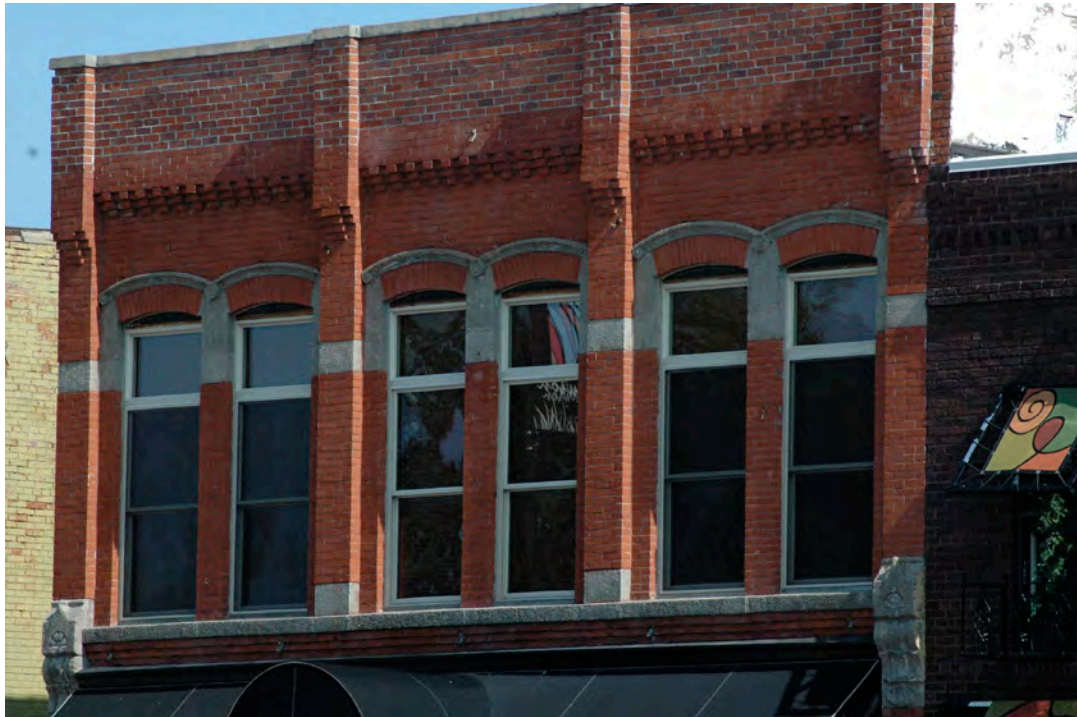
View of the upper façade. The loss of the historic cornice is unfortunate.
